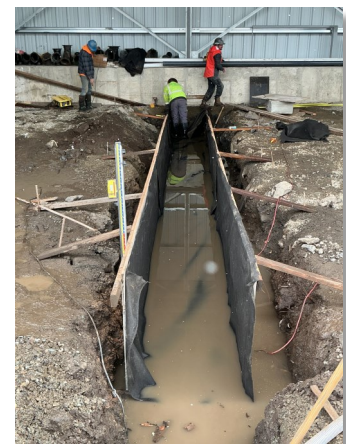
Snoqualmie Pass Utility District Phase 2 and 3 MBR WWTP Improvements
